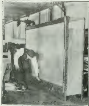
Fig. 16.—Wire-Mesh Partition Around Duplex Cutter Gears, Partition Covering all Gears.
